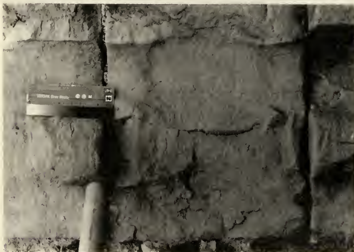
Fig. 25. Cracking and partial loss of tuff at cornice level in west wall of nave (Photo: Anne Brackin).
